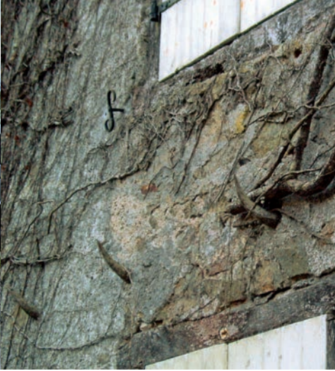
One of the characteristic features of the tanneries is still set in the wall of this house: the cattle horns which were used to stretch the skins.
