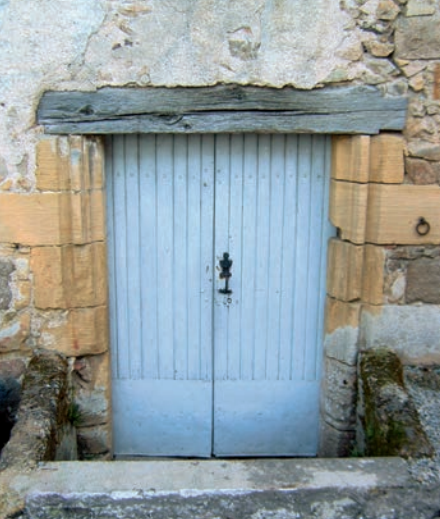
From the outside, only this door, with its abutments of Pressac limestone, reveals the existence of the Sainte-Anne chapel. Rib brackets are visible inside.
